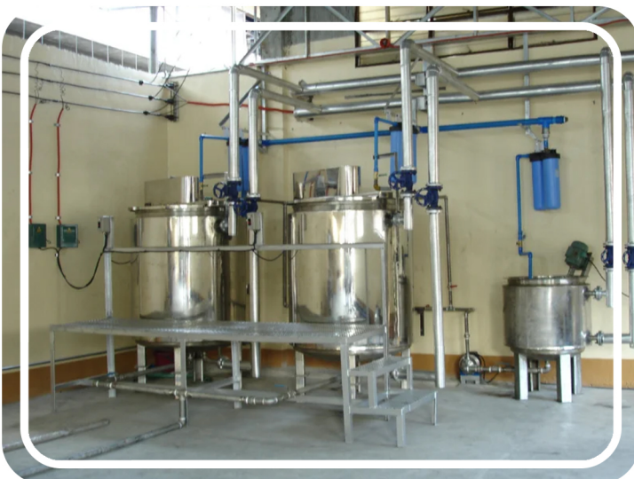
MIXER FOR BEVERAGE PROCESSING PLANT
